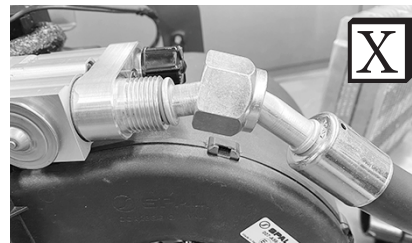
Improperly Seated O-ring Land
